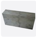
Cracked concrete ungerissener Beton
